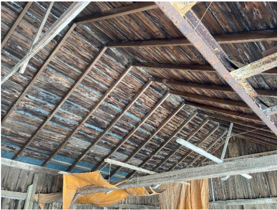
Plate 102: Interior of Outbuilding No. 1 showing rafters and plank sheathing of the roof
