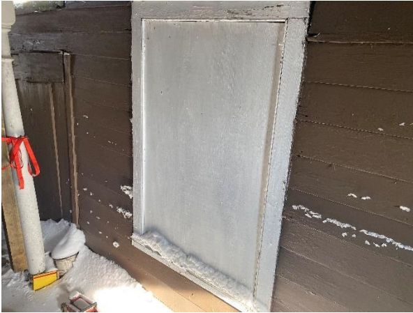
Plate 81: Framed window opening between frame and plywood addition to storage room/summer kitchen
