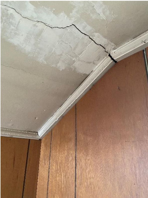
Plate 54: Cracks and repairs of southeast room
