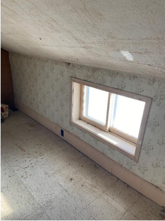
Plate 56: Detail of east knee wall or “bellyflop” window with recent trim in the northeast room
