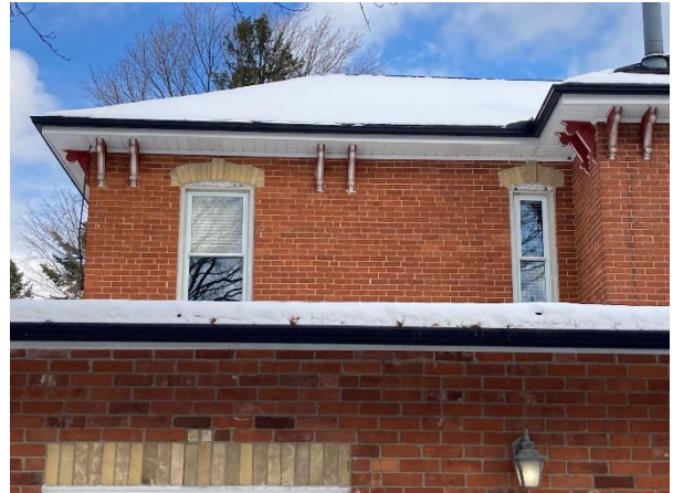
Plate 37: Upper storey windows of main block west elevation showing possible later replacements of some decorative element such as brick arch heads
