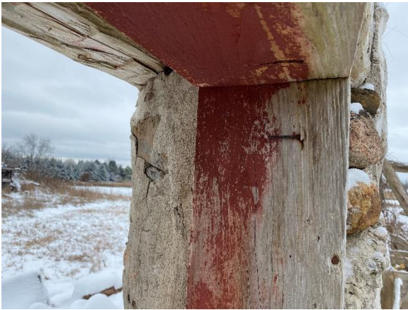
Plate 25: Wood window frame joint
