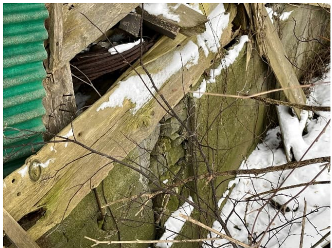
Plate 52: Delaminated concrete parging on the north elevation
