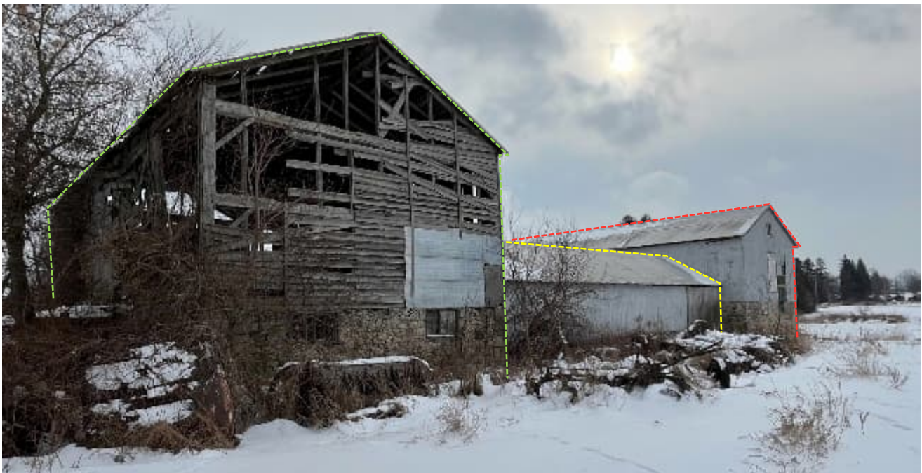
Plate 16: North and west elevations of the H-shaped barn complex (North Barn outlined in green, drive shed outlined in yellow, South Barn outlined in red)
