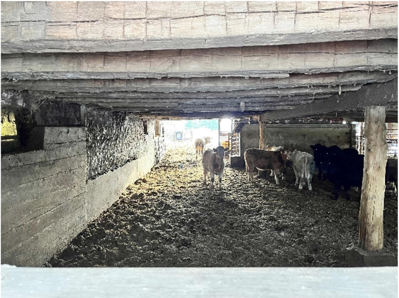
Plate 36: Lower level of the barn showing the hand-hewn beams and log posts
