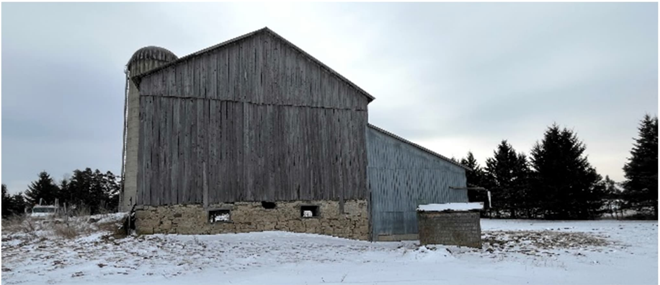
Plate 17: North elevation of Barn No. 1 (barn outlined in red, south addition outlined in green)
