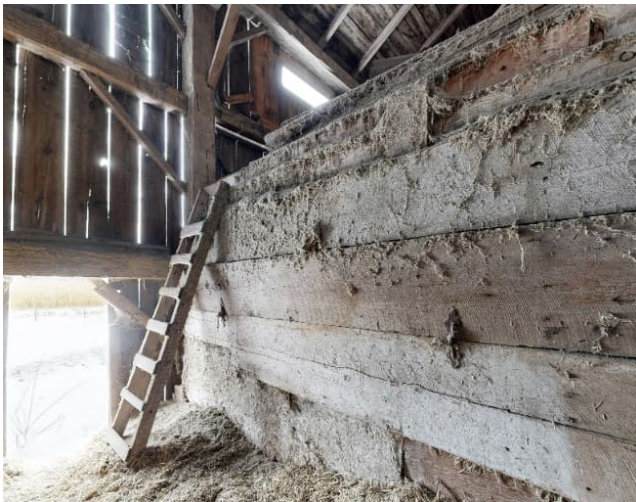
Plate 34: Looking out through the northeast entrance with ladder leading to the mow
